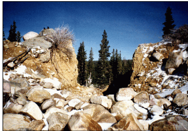
Breach in Sand Lake Dam, Carbon County, Wyoming
