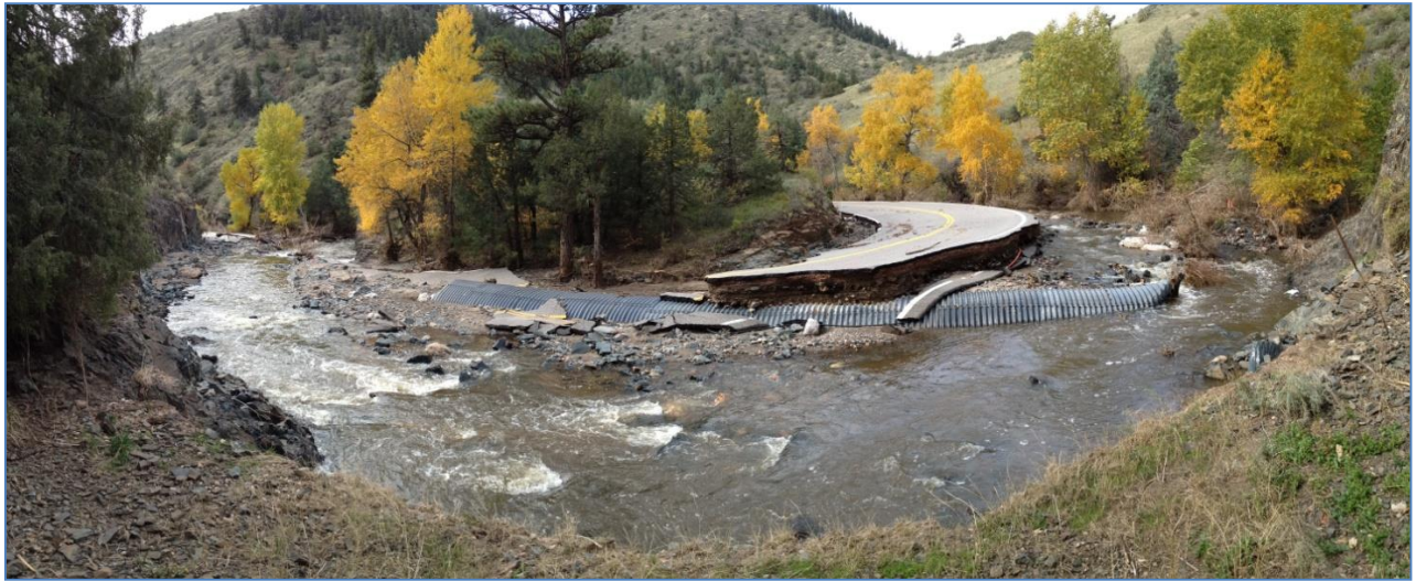
The Narrows of Larimer County Road 27 and Buckhorn Creek – Post-flood (October 2013)
