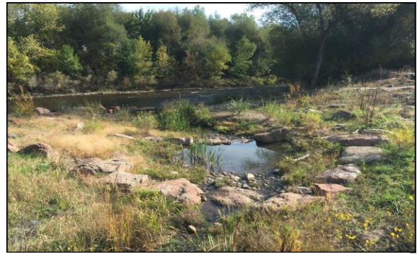
Outfall Structure at Confluence with Cache la Poudre River (After 1 Growing Season)
