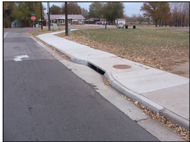
Type-R Inlet on North Impala Drive
