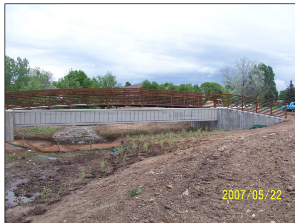
New flood control girder and pedestrian bridge at pond outlet.
