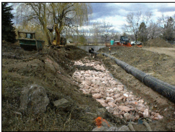
Looking Upstream at Riprap on South Bank and Temporary Bypass Pipeline in Channel.
