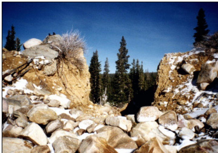
Breach in Sand Lake Dam
